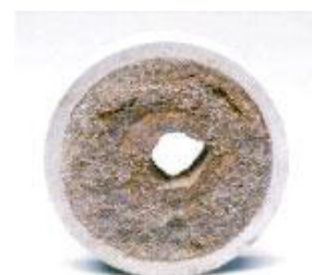
Figure 1 – Example of wax deposits in a pipe
